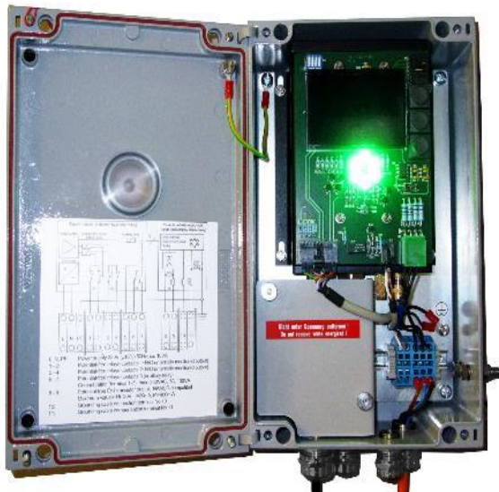
Figure 3: Configuration of EKX-4 in gas hazardous areas with opened enclosure and power switched on
